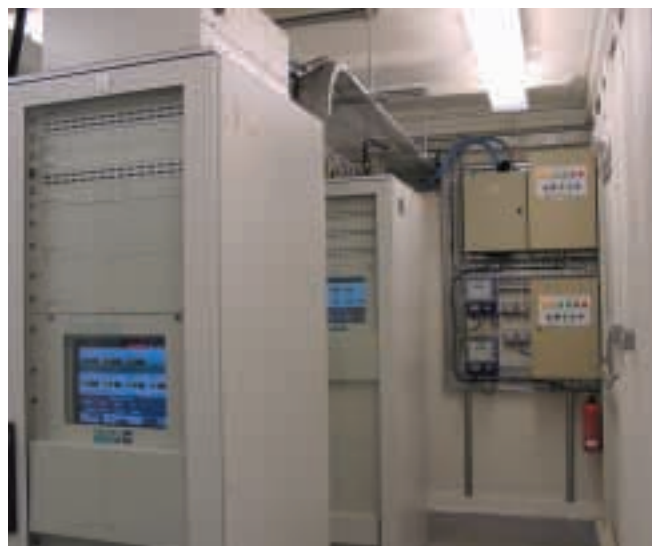
Figure 2. Multi-component extractive gas analysers (courtesy of Signal Group Ltd)
